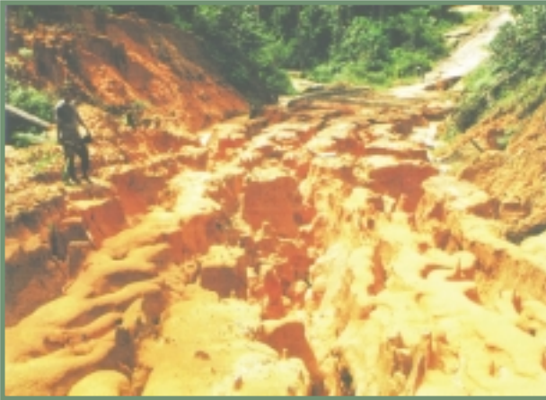
Figure 12. Heavy erosion on a poorly drained road. (Source: Critchley and Bruijnzeel, 1994)
