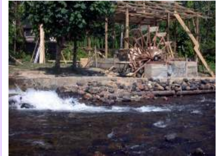
Construction of small-scale hydropower facility that allows villagers to get electricity from their stream proved to be an incentive to maintain the forested landscape mosaic intact, with its global benefits
